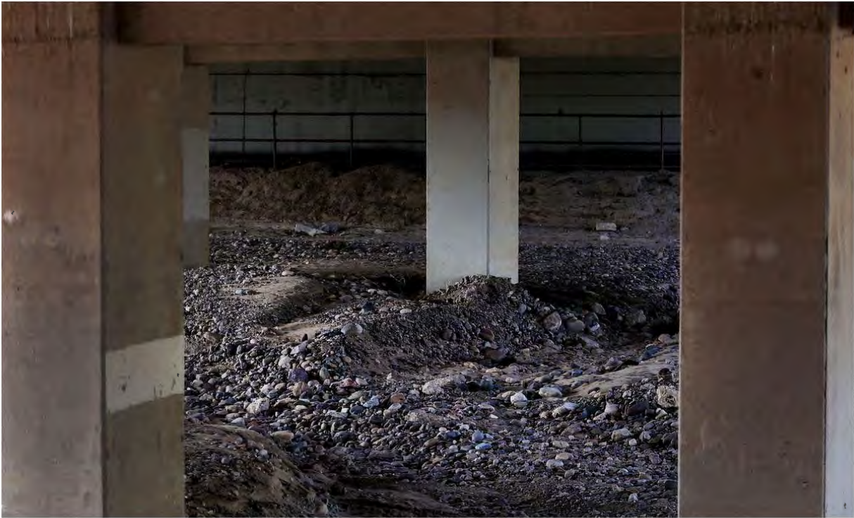
Sediment has accumulated against the concrete bridge abutments at Starr Pass Boulevard along the Santa Cruz River west of Interstate 10.
