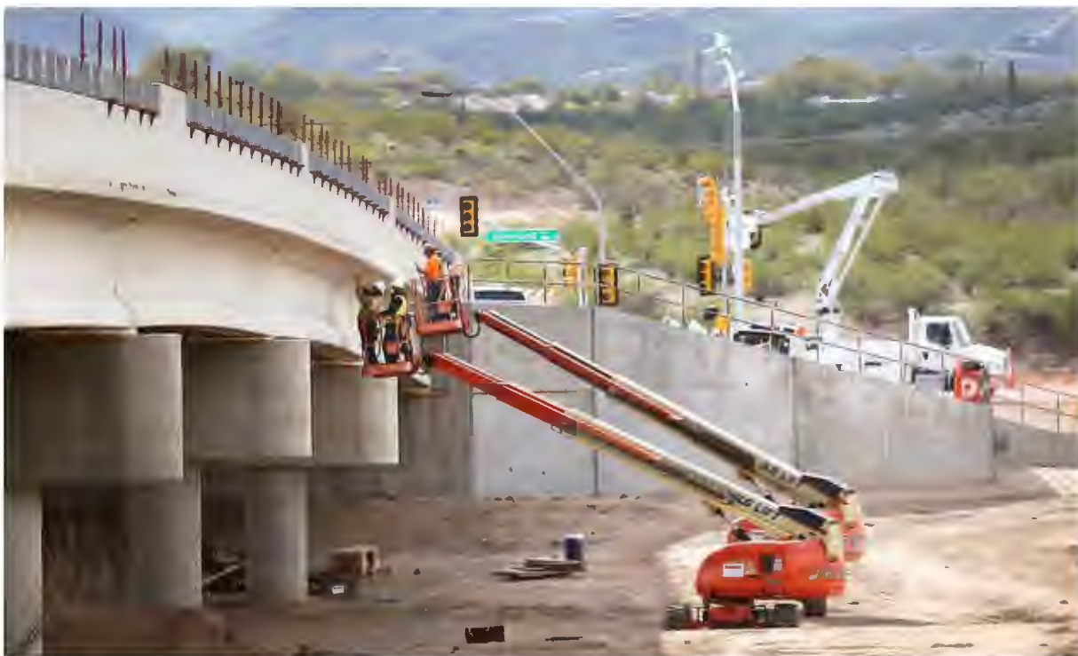
As crews work on the Sunset Road bridge over the Santa Cruz River in February, 2017. It is the newest bridge over the river.
